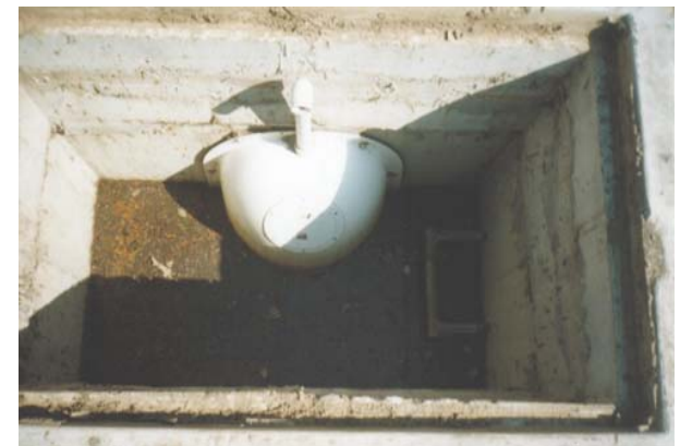
The SNOUT Trapping Floatable Oil and Debris
