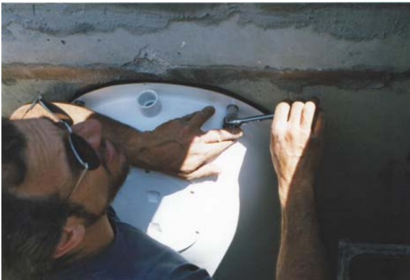
SNOUT is Bolted to Wall with Gasket on SNOUT Flange
