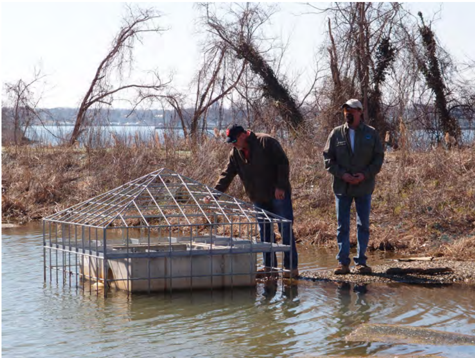
Mark Friar and a colleague inspect the water quality structure with the SNOUT and TrashScreen
